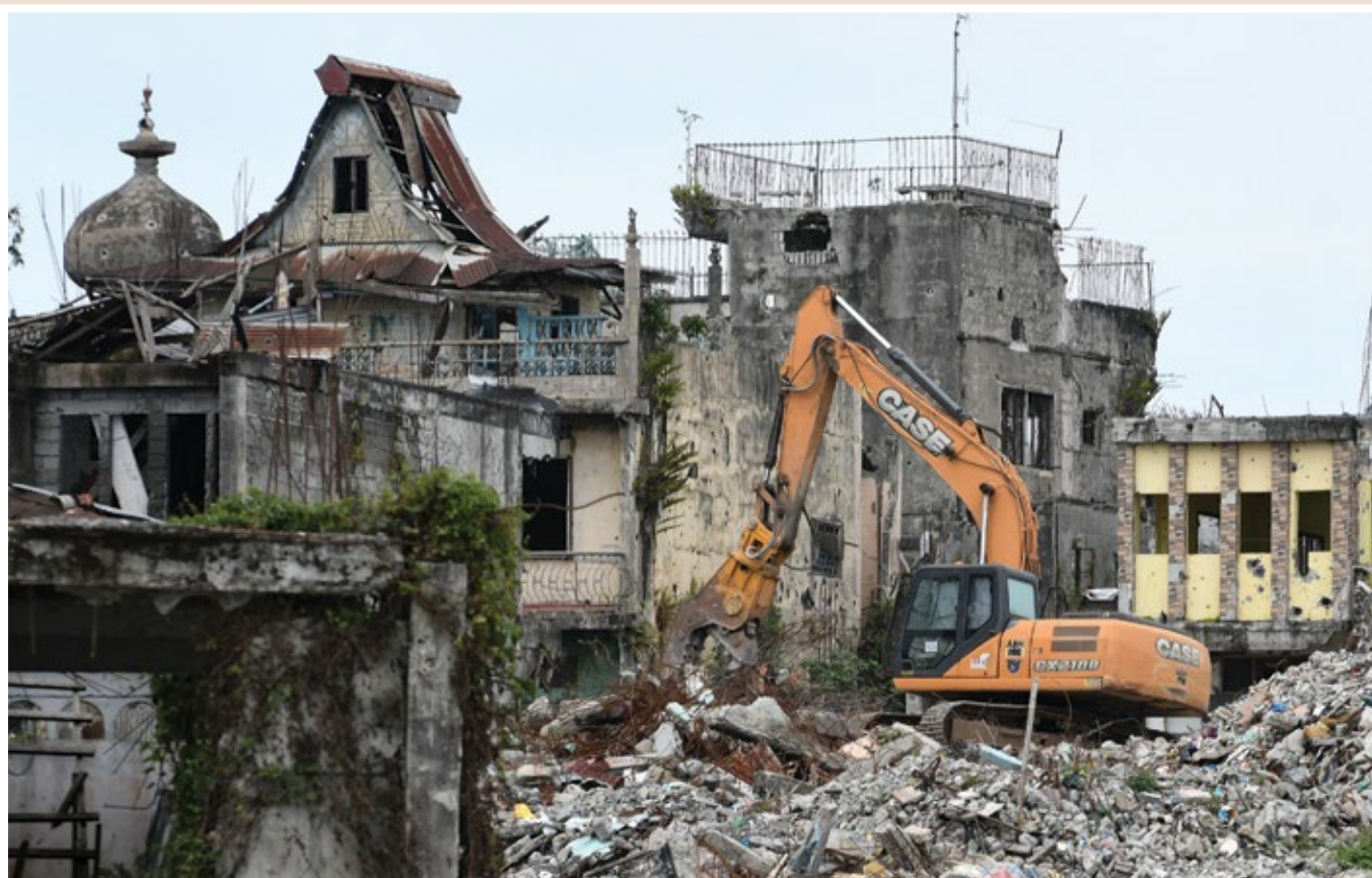
An excavator tears down buildings in Marawi City, 4 September 2019. The Task Force Bangon Marawi intensified efforts in demolishing more than 3,000 ruined buildings in the former battleground to meet its 2020 deadline for clearing the city of debris. 📷 Froilan Gallardo
